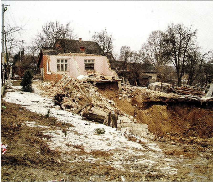
Fig. B.4. Ruined house in the area of gypsum karst (Pisky village, Lviv region, 2008)
